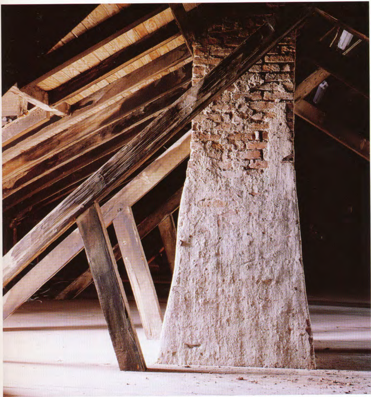
FIG. 18 BRICK AND PLASTER CHIMNEY WITH ROOF STRUTS SUPPORTING RAFTERS, MADAME JOHN'S LEGACY, FRENCH QUARTER
